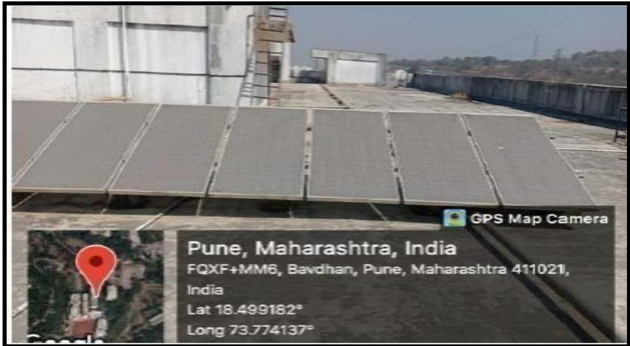
Solar panel installed on roof top of Main Building
