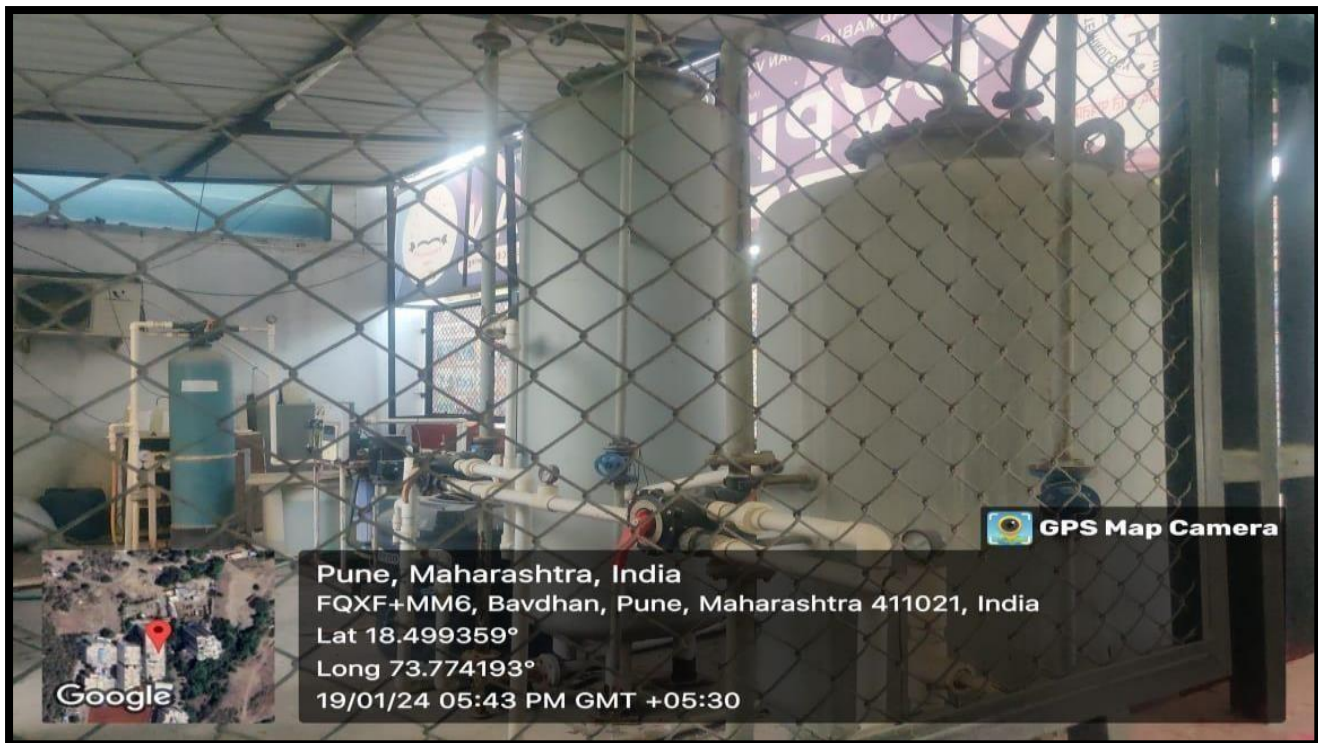
Ro Water Treatment Plants
