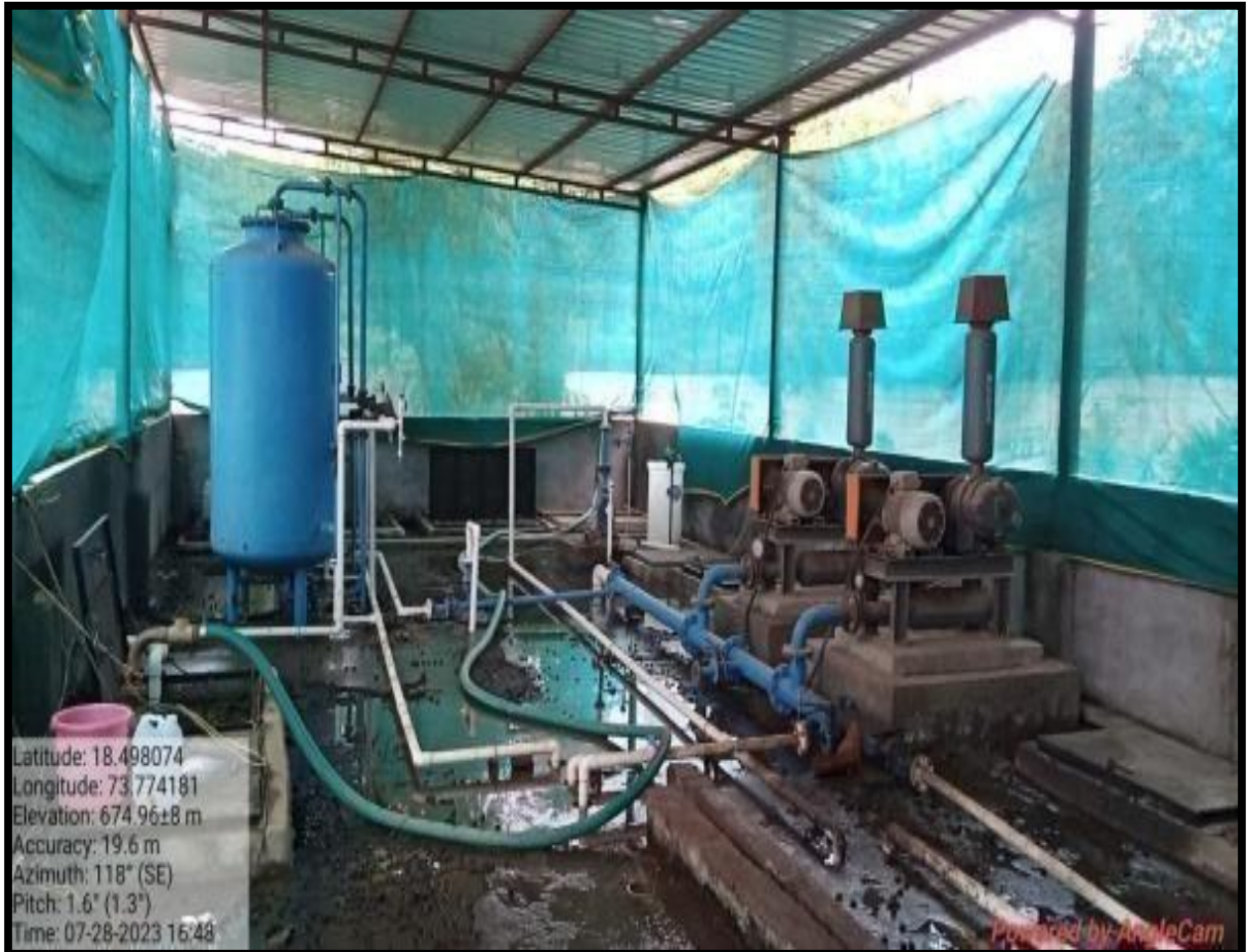
Sewage Treatment Plant for Waste Water Recycling
