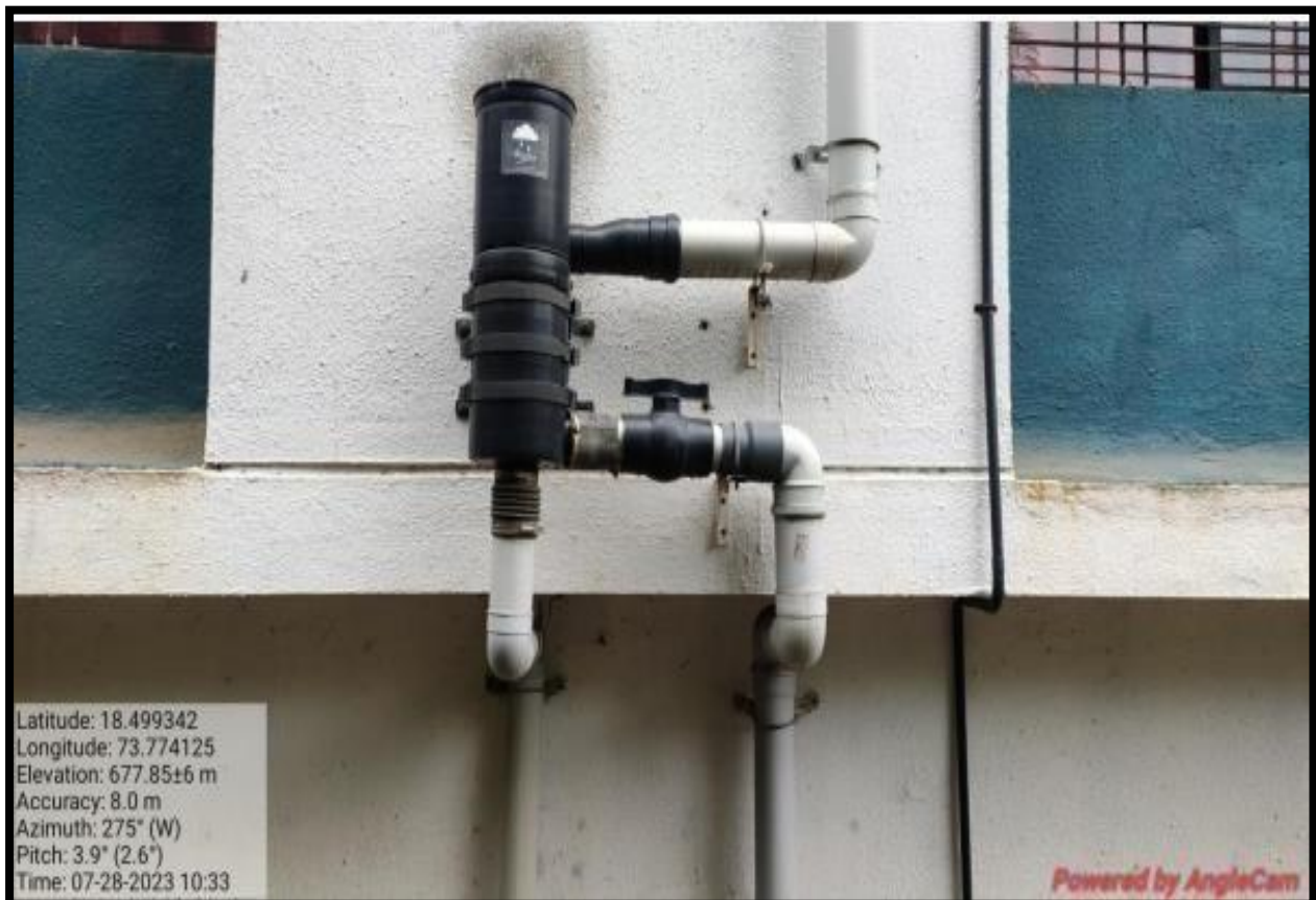
Arrangement of Rain Water Harvesting pipes from rooftop of the building to the water tank
